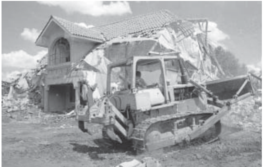
Ministry of Public Works and Housing bulldozers demolish a house on a city bypass recently. Construction of planned bypasses will help ease traffic congestion in Nairobi.
